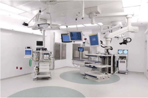
Fig. 8. Current (future) endoscopic/laparoscopic operating room. Ceiling mounted flat panel monitors. Built-in endoscopy table with adequate room for laparoscopic applications. Ceiling mounted camera for external footage. Touch panel control allowing for routing of different source images on different monitors. Wall plug in for C-arm integration with room monitors. Wall panel integrating operating room with audiovisual center allowing for video capture, integration with conference rooms, and teleconferencing. (From Duke University Medical Center, Durham, North Carolina.)
